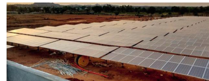
Photos: Rays Power Infra
