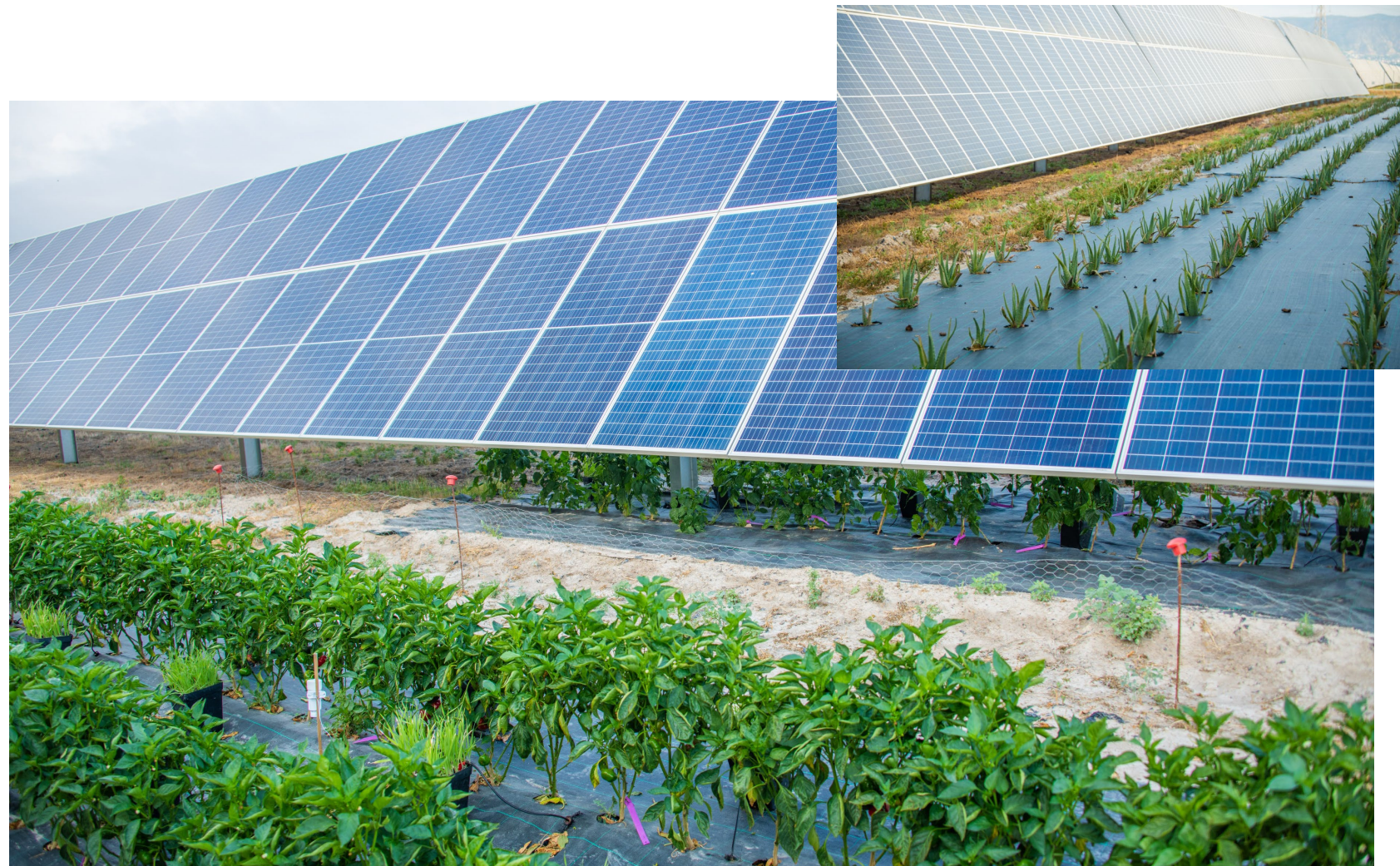
Enel Green Power's Agrovoltaic Plant
