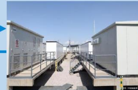
Power Booster Station AC110KV-220
