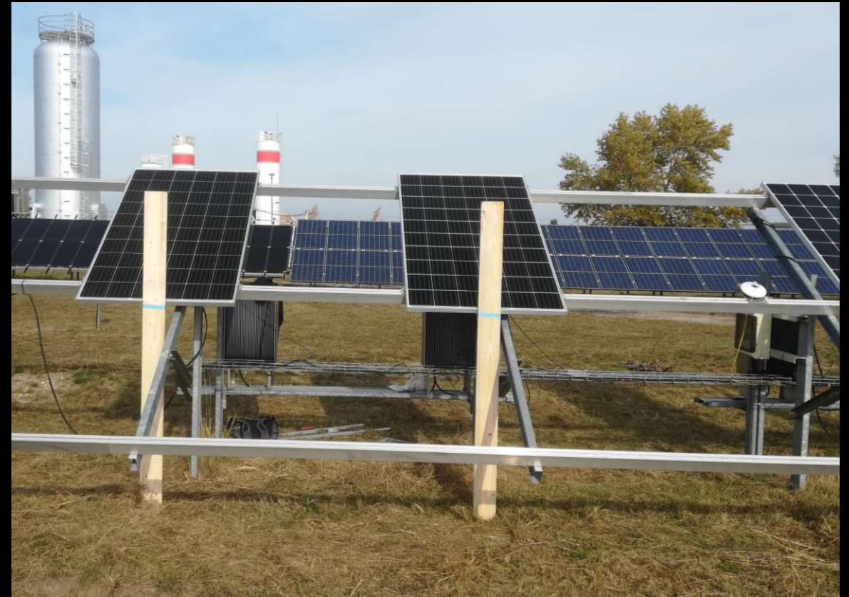
Energy yield measurement setup at the Anhalt Photovoltaic Performance and Lifetime Laboratory (APOLLO) in Bernburg, Germany
