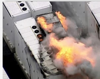
Australian energy storage accident in 2021
