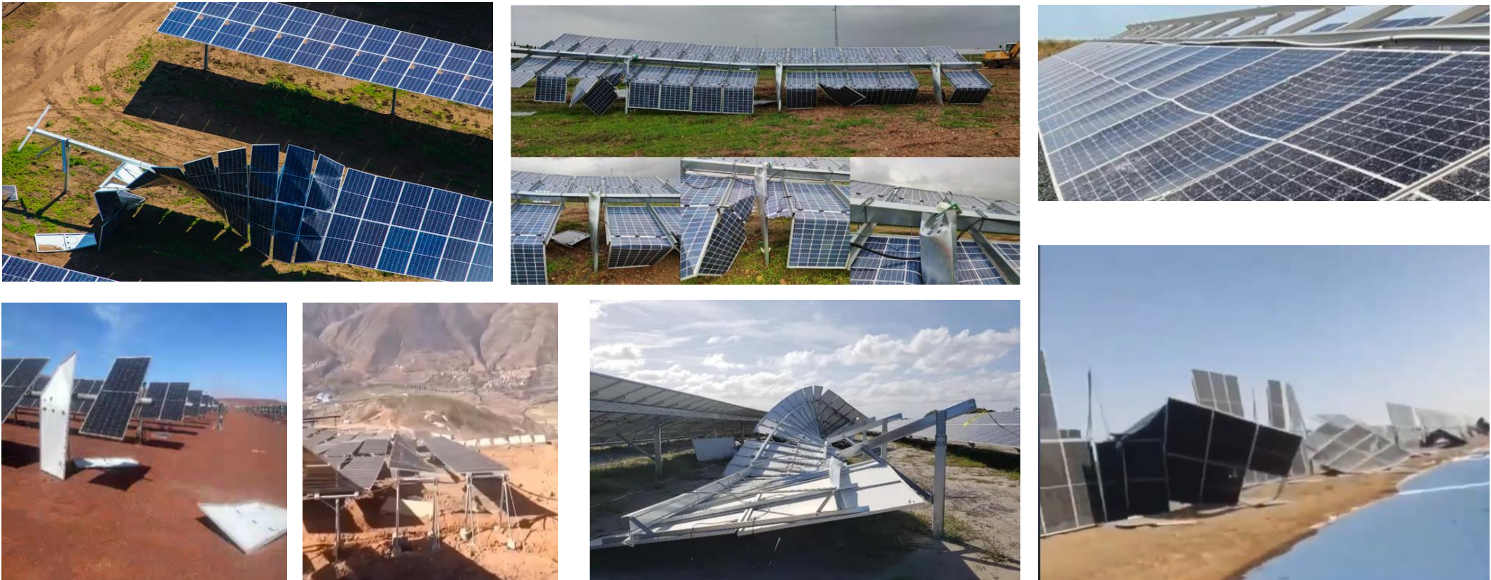
Figures: Solar mounting failures reported on social media
