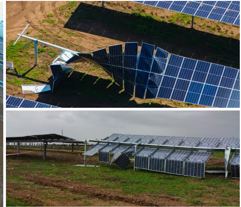
Figure: Aftermath of damage incurred:
