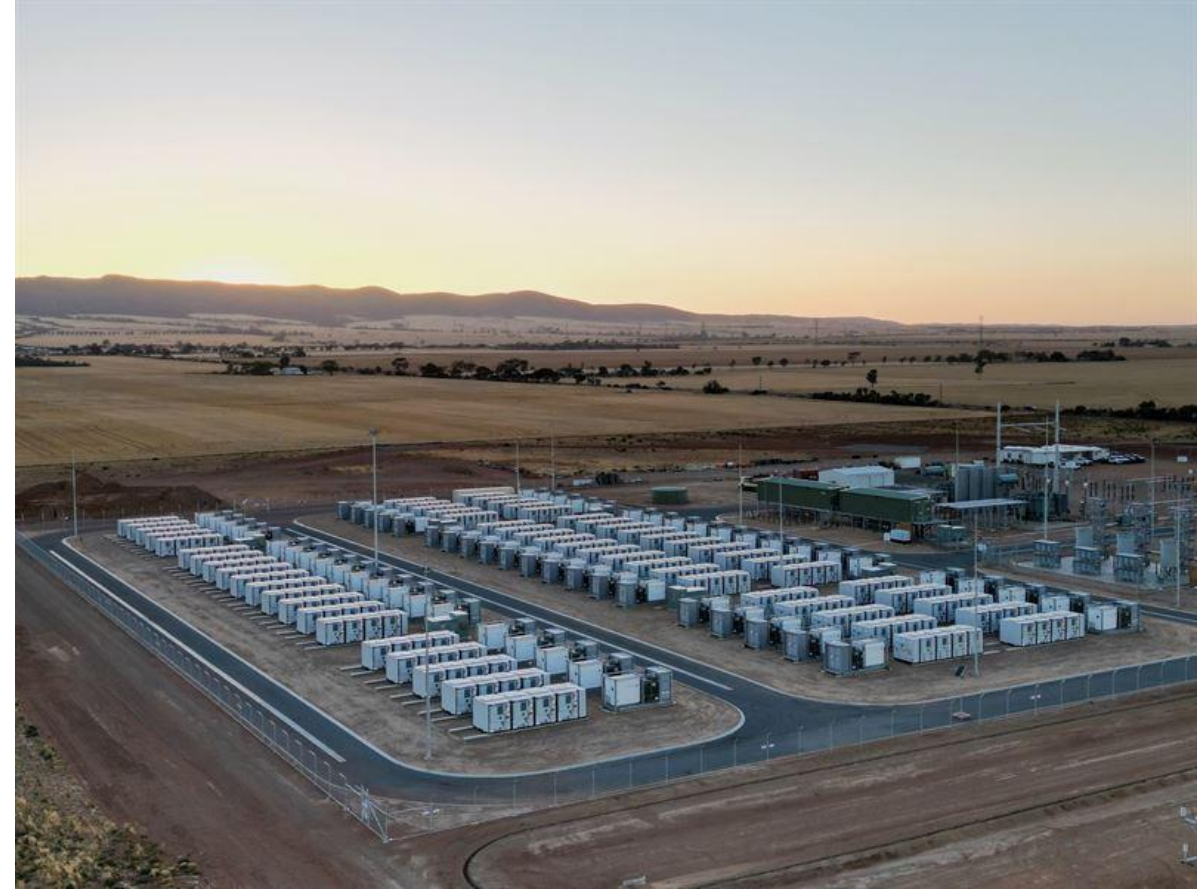
Bungama BESS Facility Online 30/06/26 - Wärtsilä
